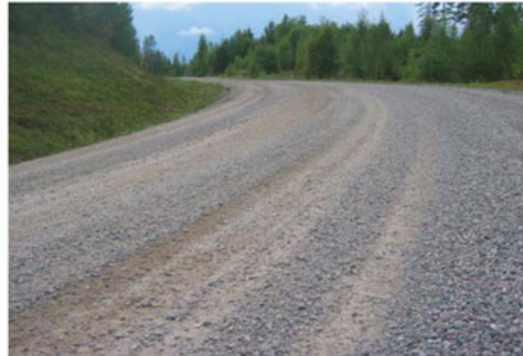
Loose gravel condition type 4.
