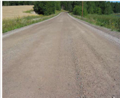
Loose gravel condition type 2.
