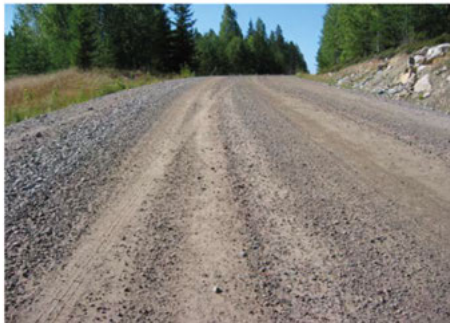
Loose gravel condition type 3.
