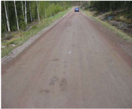
Loose gravel condition type 1.
