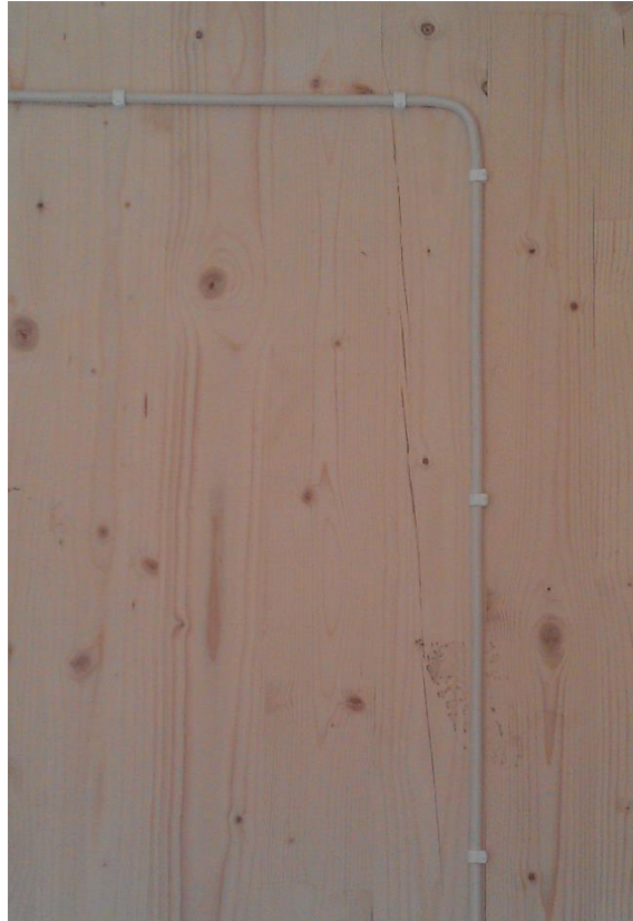
Figure 12. The picture shows cracking in a CLT panel approx. five months after the assembly of the building. However, thermography in connection with pressure testing shows no sign of this cracking causing any extra air leakage, partly because the CLT panel is built up of several layers.
