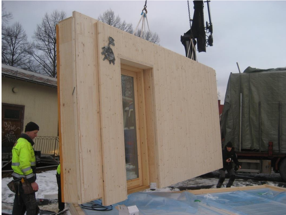
Figure 14. Assembly of the north wall. The position of the lifting loops means that the wall leans somewhat which makes placing it on the floor element more difficult.
