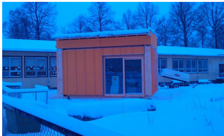
Figure 3. Test building in the twilight the day after the assembly. The joints between the wall and roof elements remained to be completed as did the external boarding.
