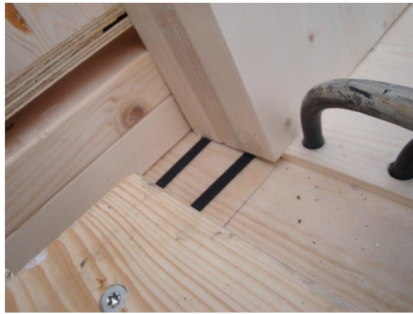
Figure 13: During assembly the wall elements got stuck on the edge of the reveal in the foundation element.
