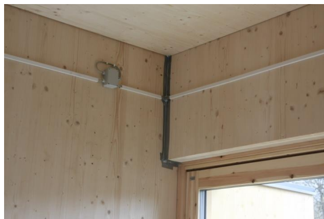
Figure 25: Temporarily sealed joint in the elements above the sliding door screen. This joint has not been sealed during the recurrent air tightness tests.
