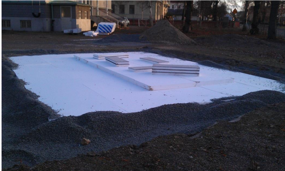
Figure 2. The foundation of the test building before the CLT panels have been laid. The cellular plastic boards with fibre cement cladding which are laid over the foundation are to hinder the cellular plastic boards from being blown away.
